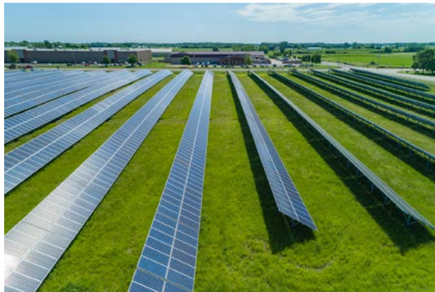
EXAMPLE OF A SOLAR PROJECT IN OPERATION
