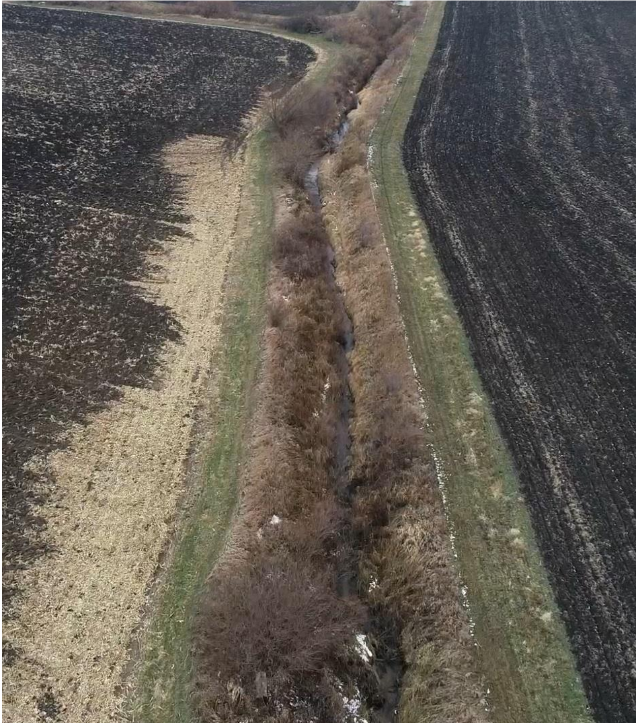
Photo 2: Vegetative debris that has accumulated upstream of Station 30+00 culvert.
