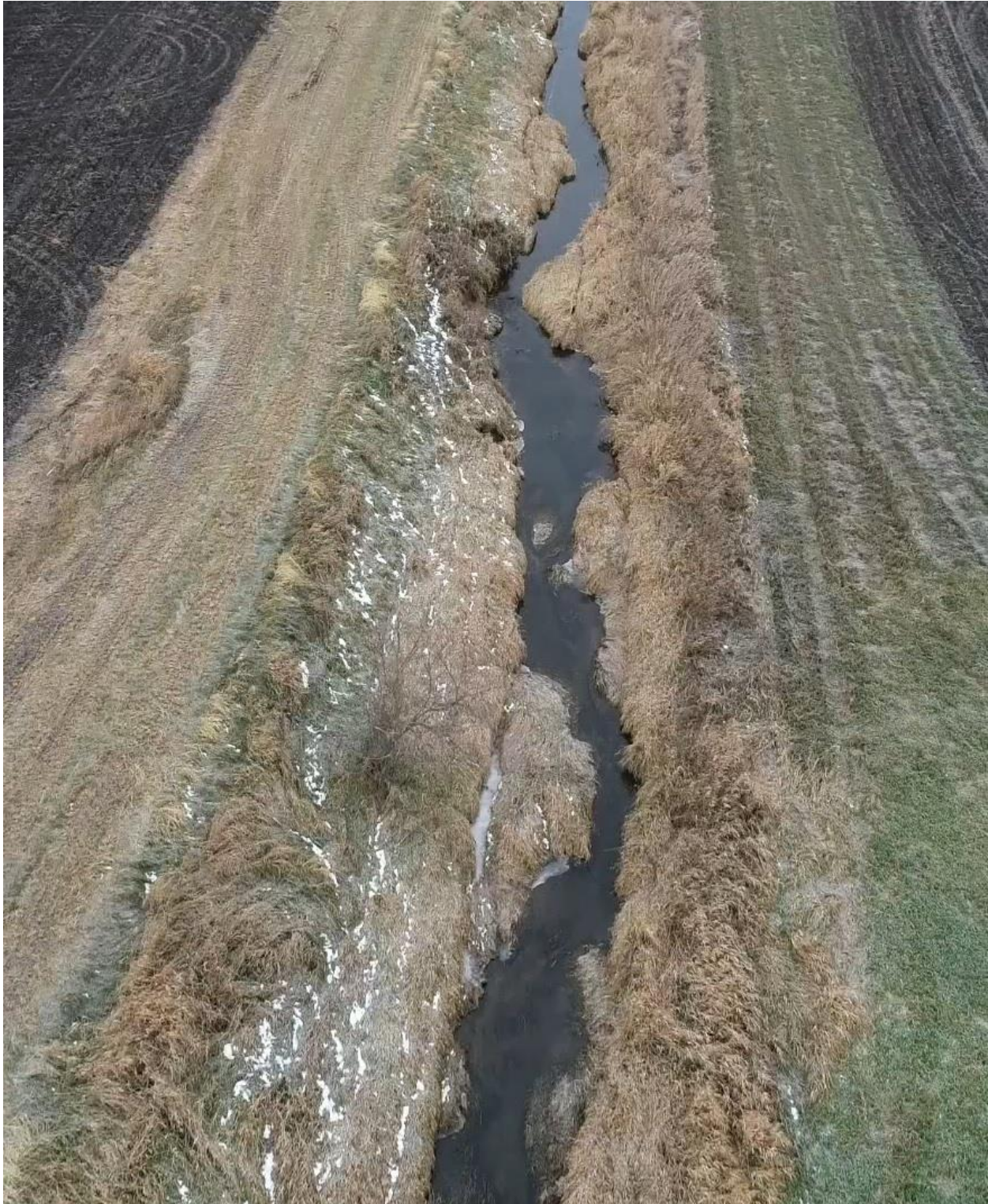
Photo 3: The banks of the ditch are sloughing, likely due to the meandering ditch channel.
