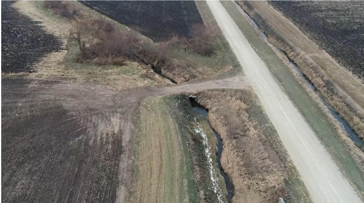
Photo 5: The CMP culvert at Station 30+00 is in disrepair.
