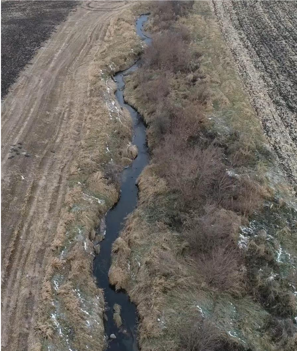
Photo 4: The banks of the 10-foot wide section are sloughing, likely due to channel meandering.
