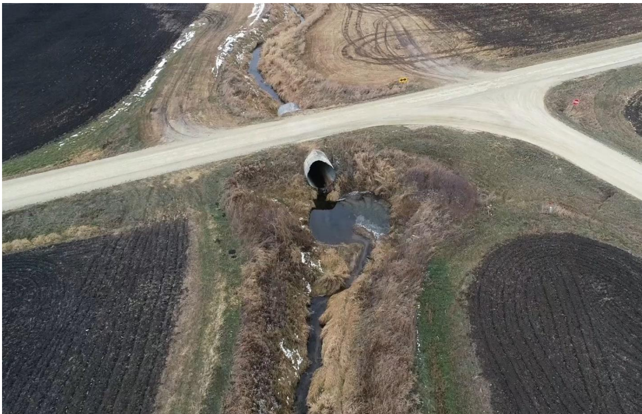
Photo 6: The CMP culvert at Station 60+72 appears perched above the channel bottom.
