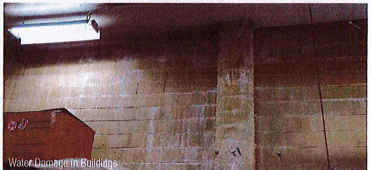
Water Damage in Buildings
