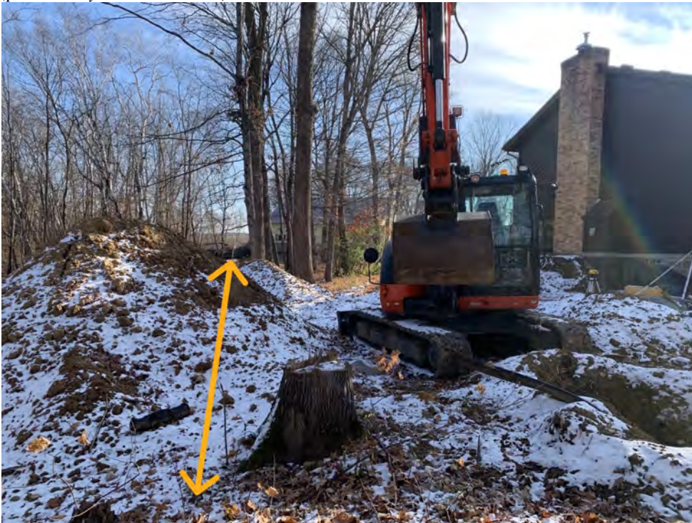
Figure 3: North Side of House, showing project area with an approximate section line drawn for reference. (provided by William Lenzen)
